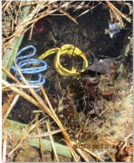
Control box full of water
