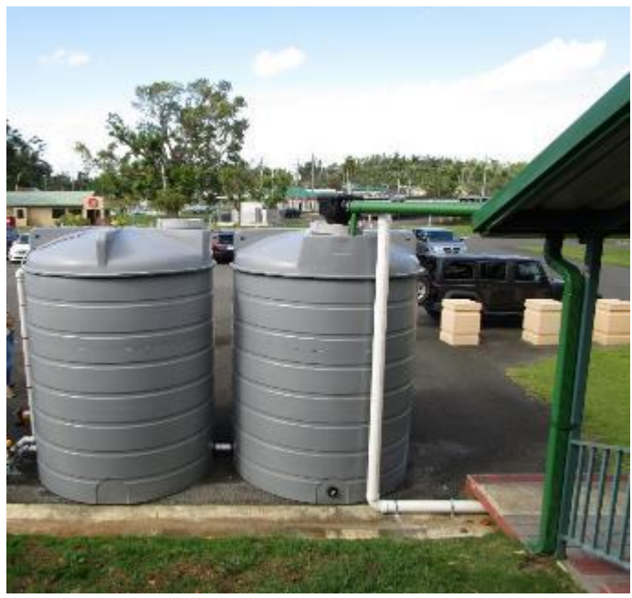
Fort Buchanan Potable Rainwater Harvesting
