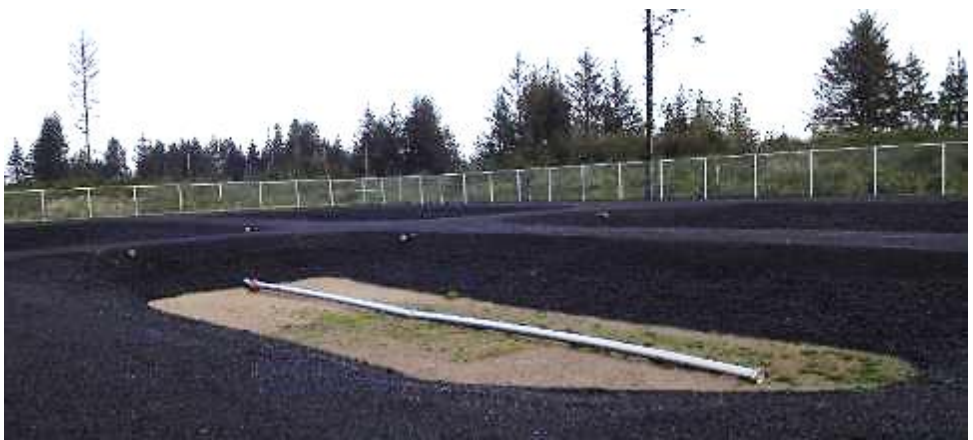
Camp Rilea Indirect Potable Reuse
